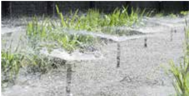
A Neptun-type filter where water is sprayed over and seeps through gravel.
